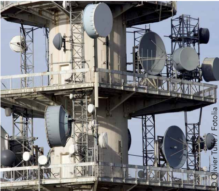
Telecom - Data infrastructure
